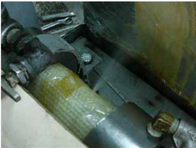
Fig.6: Leakage of inner oil through crevice in reinforced layer.
